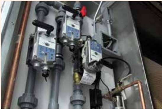
Industrial control valves
