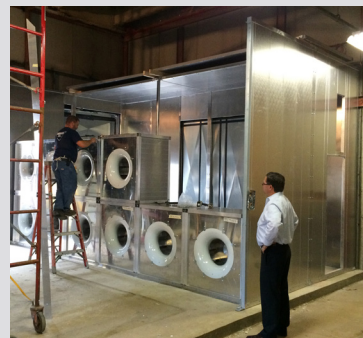
FANWALL Cubes being installed in Knock-down Air Handler on the job site
