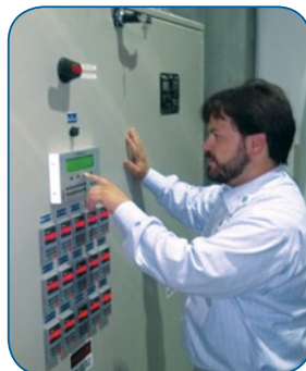
Dan Maples monitoring FANWALL airflow with the SOC DDC controller and airflow monitoring panel.
