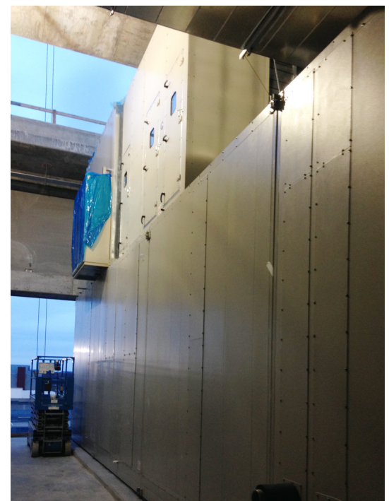
One of the two large Ventrol heat recovery units being installed during construction
